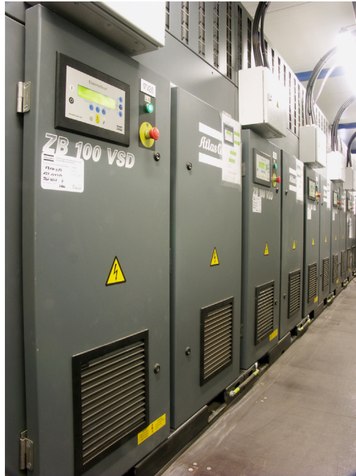
Fig. 1: The container with the six compressors arranged right next to each other was designed especially for Weser-Metall by the project department at Atlas Copco. At the end, the complete “machine house” was brought in through the building covering with a crane.
