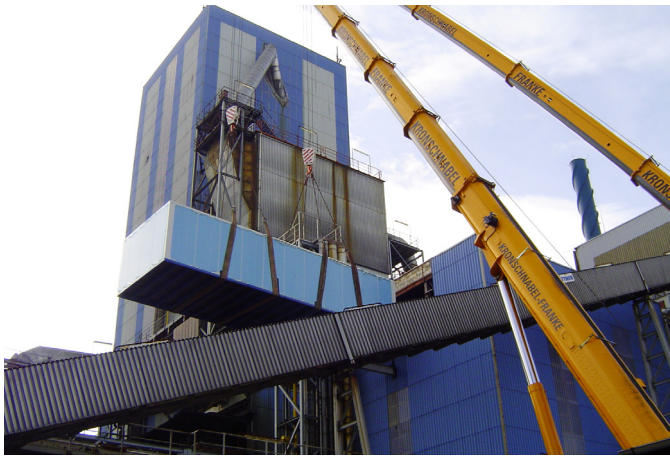
Fig. 5: Logistical master achievement: two cranes working together in order to bring in the complete compressed air station in their container-like housing through the building covering onto a platform at a height of 14 m above the old compressor installation.
