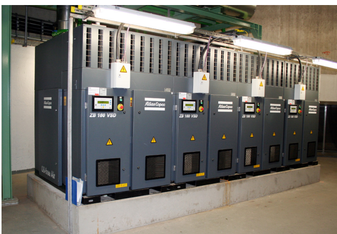
Fig. 2: Four of the innovative ZB low-pressure centrifugal compressors from Atlas Copco ensure the oxygen requirements of the new cascade basins in the Currenta waste water treatment plant in Leverkusen. Depending on the degree of contamination of the waste water, two or three run around the clock; the fourth serves as contingency reserve. Centrifugal compressors are single-stage, speed-controlled type ZB 160 VSD machines. The motors have a contactless electromagnetic bearing system, so they operate wear-free.
