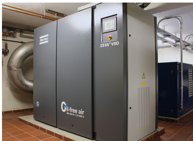
Fig. 2: Compressor station for the seepage water treatment installation. In the foreground, the new speed-controlled screw blower ZS 55+ VSD, which already runs significantly more efficiently than rotary lobe blowers due to their design.
