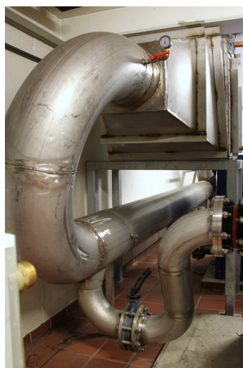
Fig. 4: Pipeline to aeration basins. The ZS blower provides the bacteria with up to 1680 m 3 of air per hour
