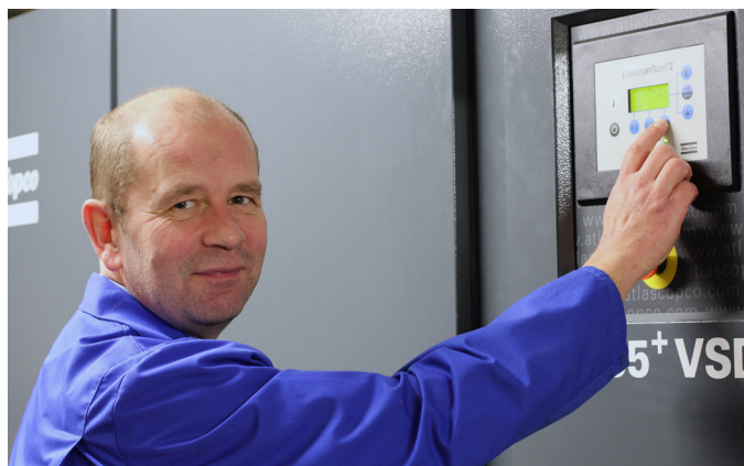
Fig. 5: Wilfried Rasch, specialist in sewage technology, helped set up the seepage water treatment installation and checks the air quality daily in the basins, as well as the performance of the compressors.
