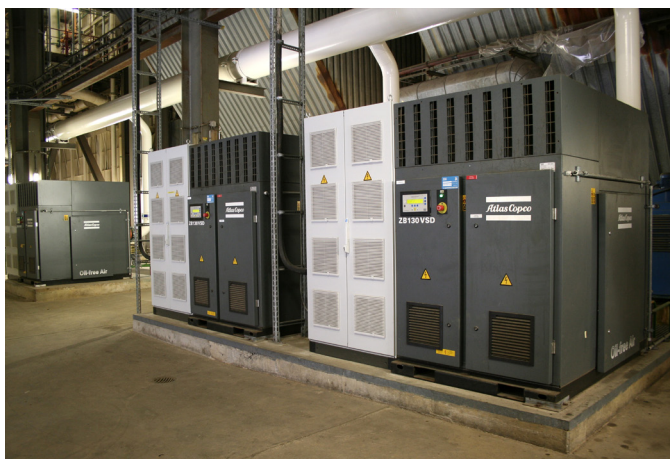
Fig. 2: Three type ZB 130 VSD speed-controlled low-pressure compressors by Atlas Copco produce oxidation air for flue gas desulphurization installation in the Ibbenbüren power plant. Power consumption has dropped by 18.1% compared to earlier.
